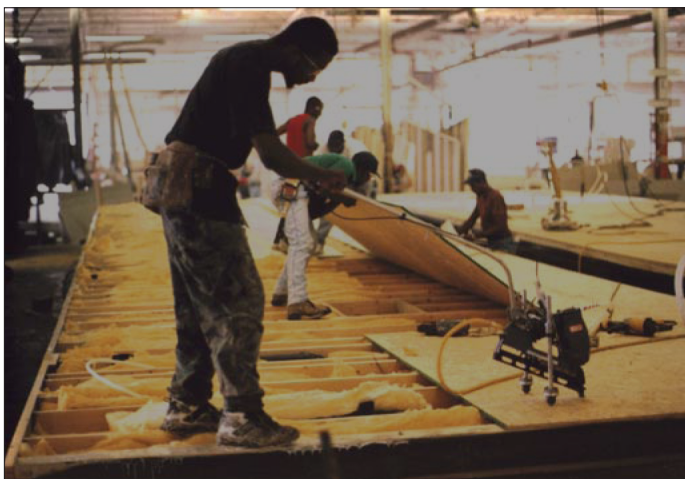
Figure 1. Reducing the risk of back injury and fatigue during nail gun operation using wheels and extensions.
