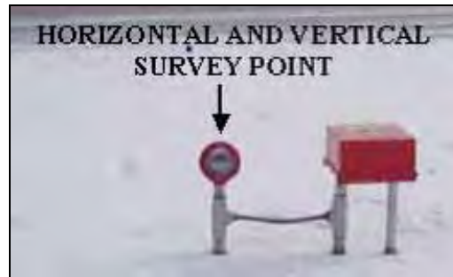
Figure C-4. Typical installation of the runway end identification light (REIL) with the horizontal and VSPs identified.
