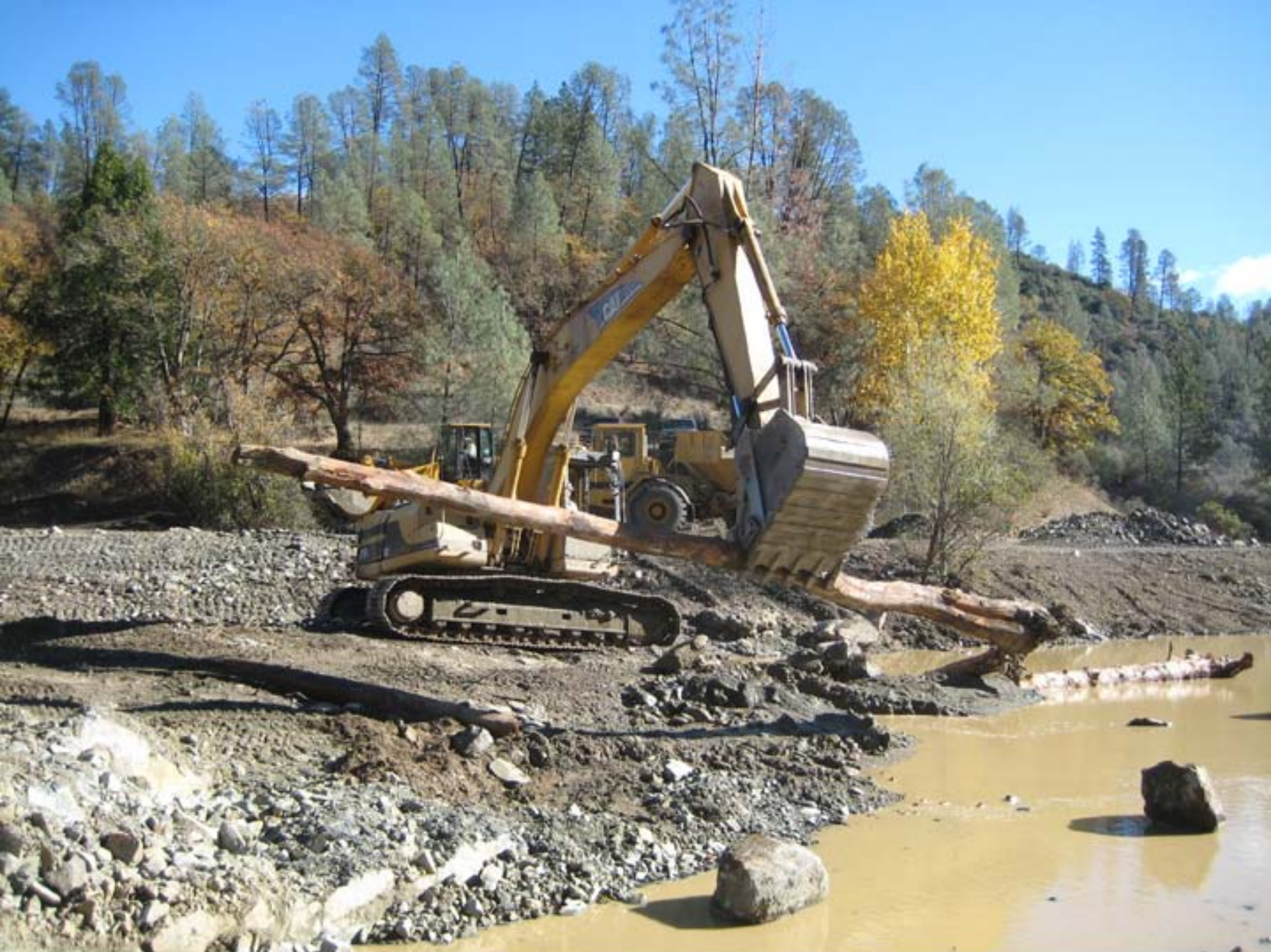
An excavator places tree trunks into an excavated side channel watercourse intended to house juvenile salmon after they hatch from gravel in the adjacent river at the Sven Olbertson salmon habitat restoration site.
