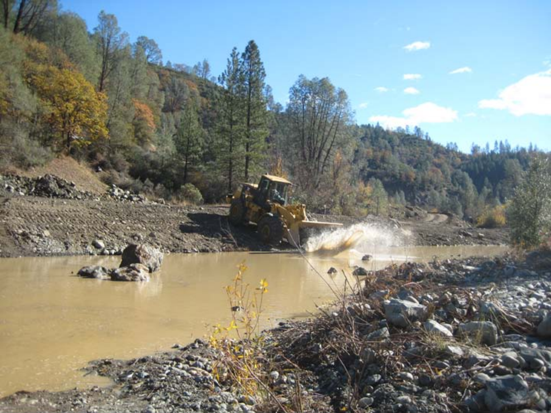
A front-end loader drops a load of boulders into an excavated side channel at the Sven Olbertson salmon habitat restoration site.
