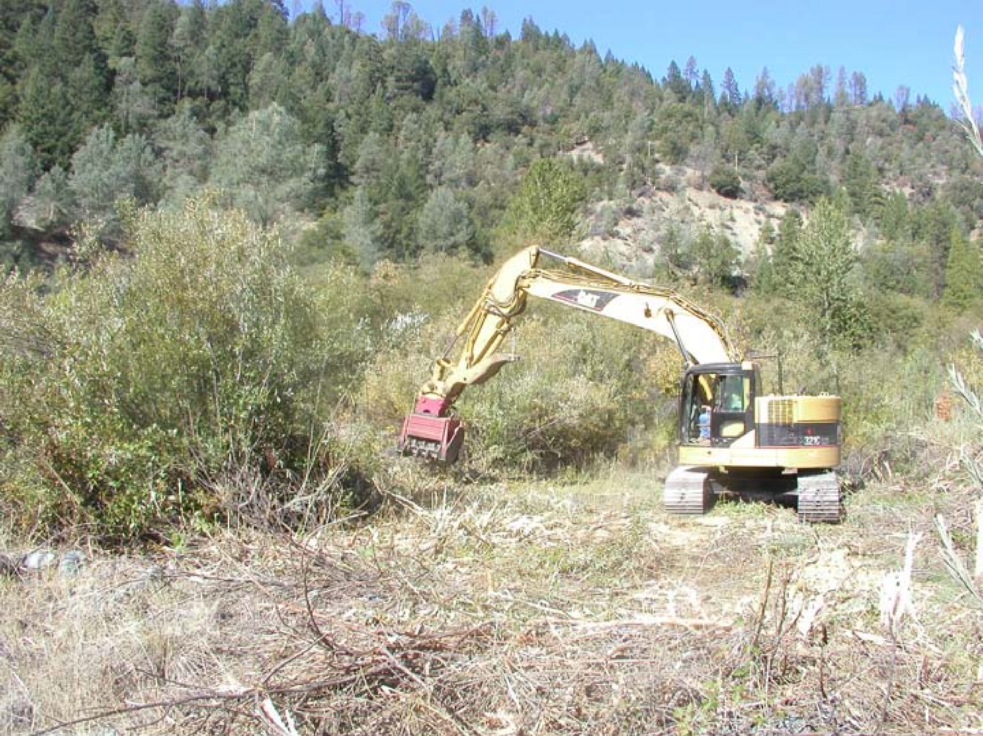
An excavator with an attachment called a masticator prepares to grind small trees and shrubs into mulch at the Sven Olbertson salmon habitat restoration site.
