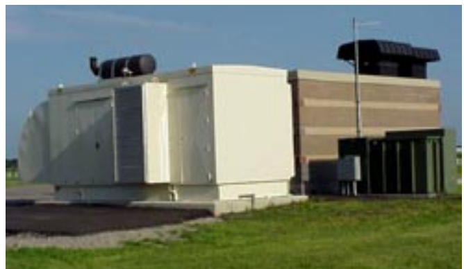
A backup generator enables this lift station (brick building) to operate during a power outage.
