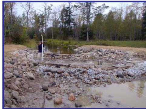
-USFWS photo by Susan Wells Potagannissing Dam on the Potagannissing River, within three miles of the Harbor Island NWR in Potagannissing Bay, was replaced by a series of rock weirs to reduce slope and provide resting pools for migrating fish.
