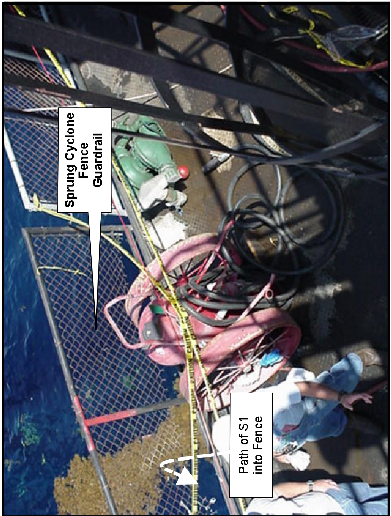
Guard Rail Opposite Manway Hatch, LLPS, after Explosion S1 Summer Wet Oil Tank Worker
