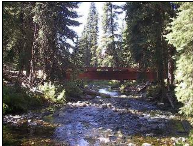
Figure 40 - Picture of Moose Creek Bridge, taken from old road prism location looking downstream.
