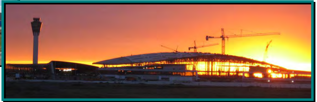
The new ARFF Facility and Terminal Building under construction at Indianapolis International Airport.
