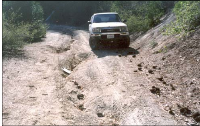
Figure 2: In 2002, Road 22N25 on Feather River Ranger District exhibits severe rutting as a result of a poorly drained surface that concentrates runoff. This road was reconstructed in 2003
