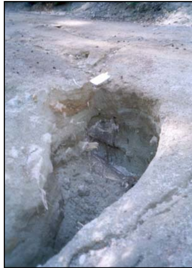
Figure 4: This bank erosion occurred on 22N25 during a normal precipitation year when concentrated surface drainage left the road at an inopportune location. The slump material was delivered to the RCA of Pinchard Creek, which is located less than 150 feet from the road. This road was reconstructed in 2003. (clipboard is shown for scale)
