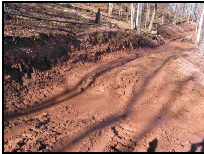
Figure AR-4. Skid Road Soil Disturbance in Day South Harvest Unit #2
