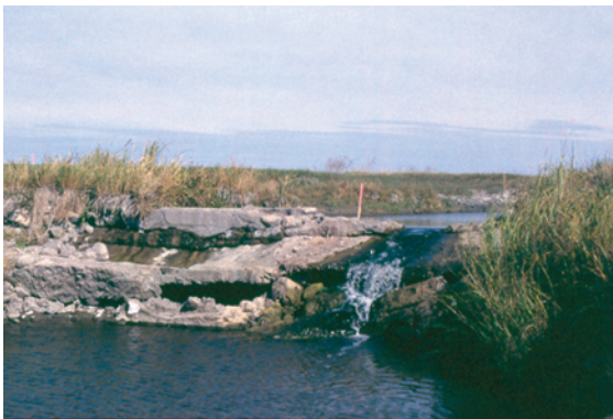
Several water management structures need repairs.
