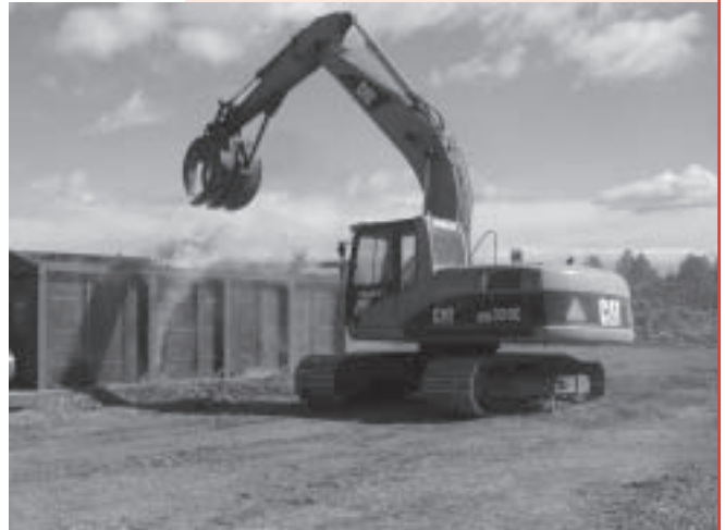
A crane loads wood debris into an air curtain destructor. The units often operated round-the-clock to take advantage of favorable air quality and burning conditions.
