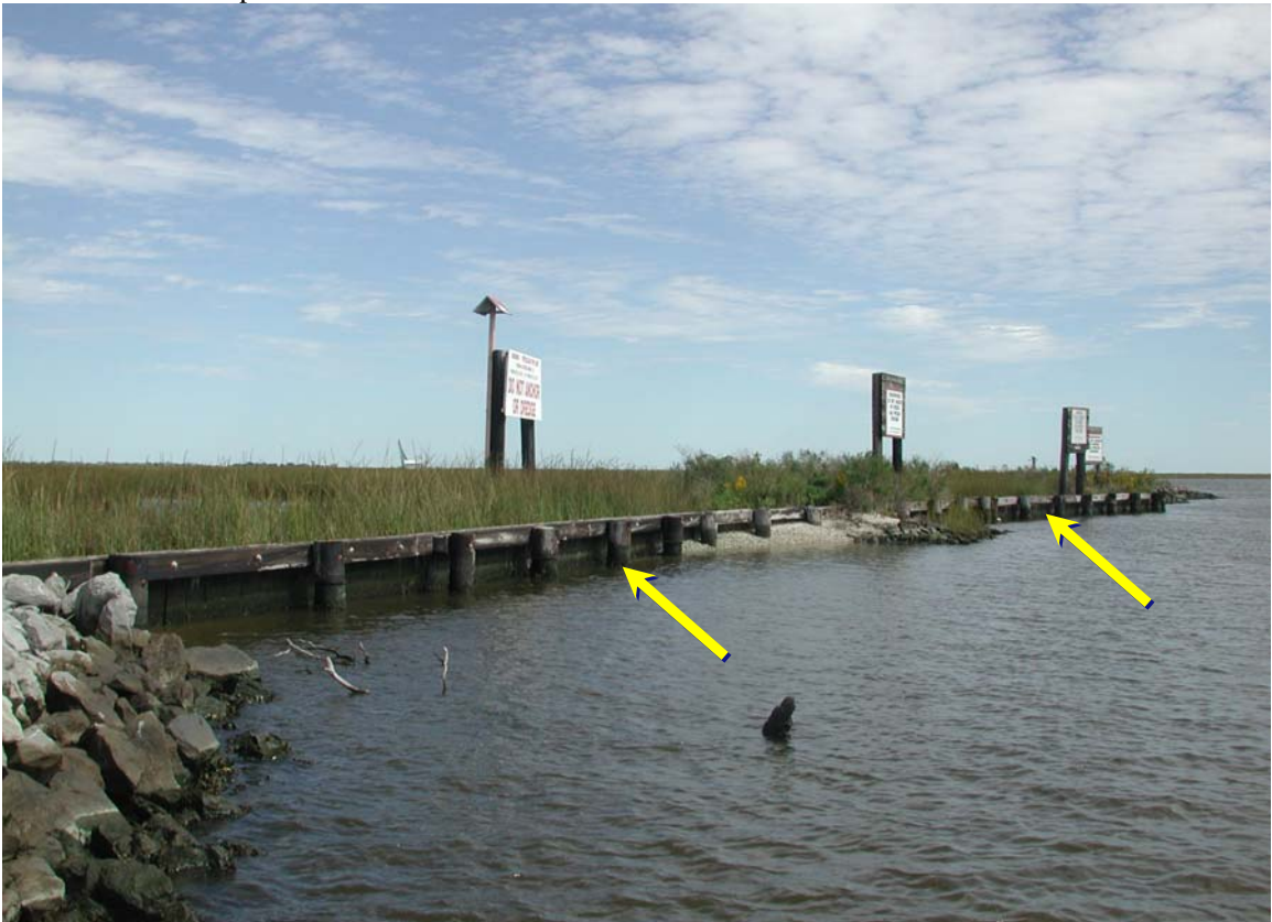
Figure 13-d. Ground photograph (October 2003) of a seawall that is part of a structure to plug a pipeline canal. In this case, there is salt marsh behind the seawall. Seawall and riprap often intermixed along developed areas
