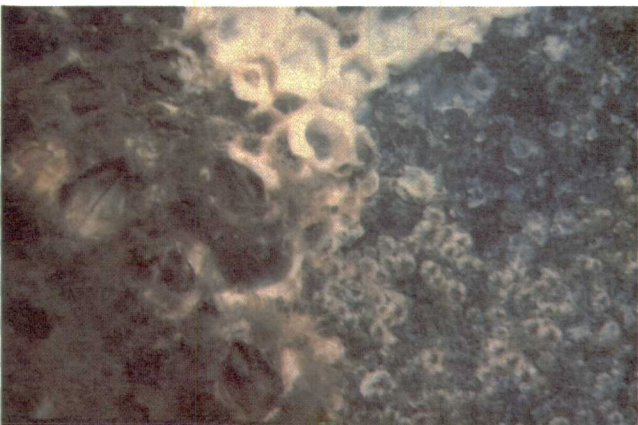
Representative barnacle dynamics at Bay Marchand 3KN; clockwise starting at upper right corner, (1) bare pipe, (2) recent set, (3) mature barnacles, and (4) grazed barnacles.
