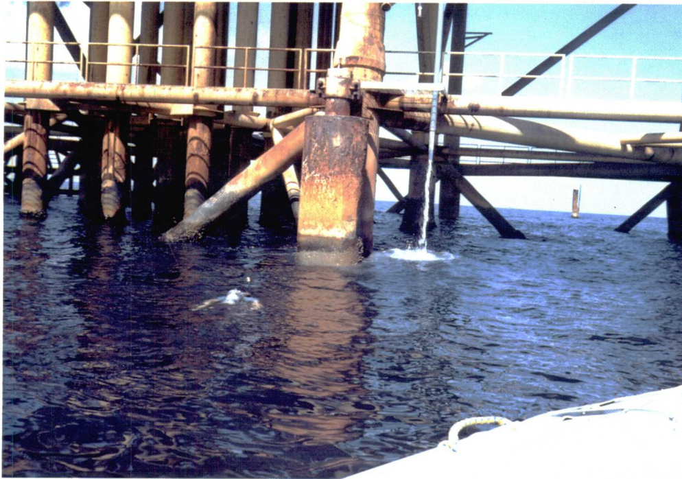
Produced water discharge just above surface.
