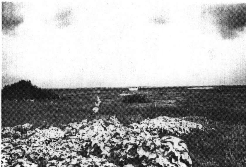
Figure 7.4. Condition of T5 and T6 ROW north of GIWW. Note bulkhead on lower right and valves on upper left of photos.
