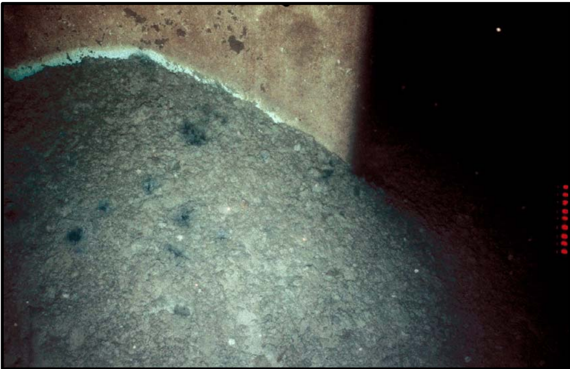
Photo 2-4 - Muds and cuttings accumulation near the base of a Ewing Bank 305 platform leg. Vertical relief of the accumulation was approximately 0.3 to 0.6 m (1 to 2 ft).
