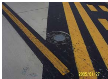
Figure 2. Photograph of in-pavement REL fixture at runway hold line.
