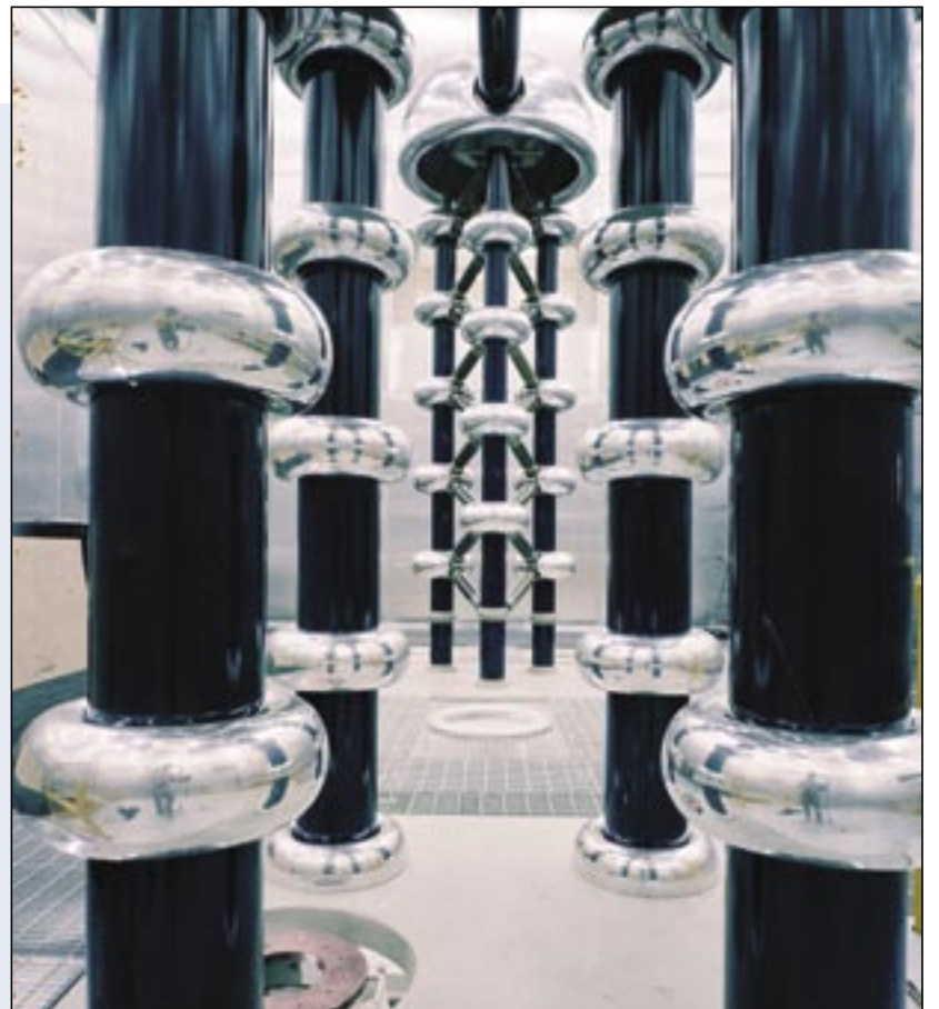
Protons at the Los Alamos accelerator begin their journey here, in the domes at the top of three of the Cockcroft-Walton accelerators. By the time the particles leave this section, they have been accelerated to 7,440 miles per second (4 percent of the speed of light). From here, the beams pass through low-energy transport systems where they are steered, focused and bunched for injection into the second stage of the accelerator. File photo
