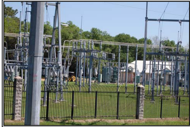
It all starts here: Tallahassee substation #31.
