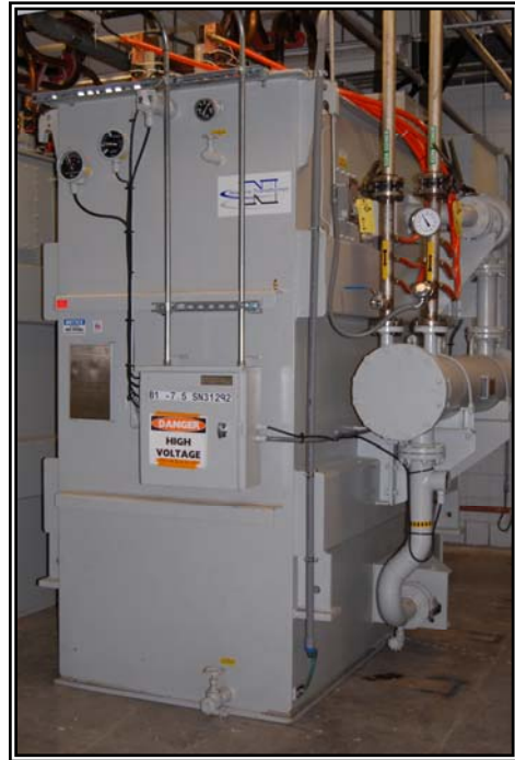
One of the 28-ton transformers.
