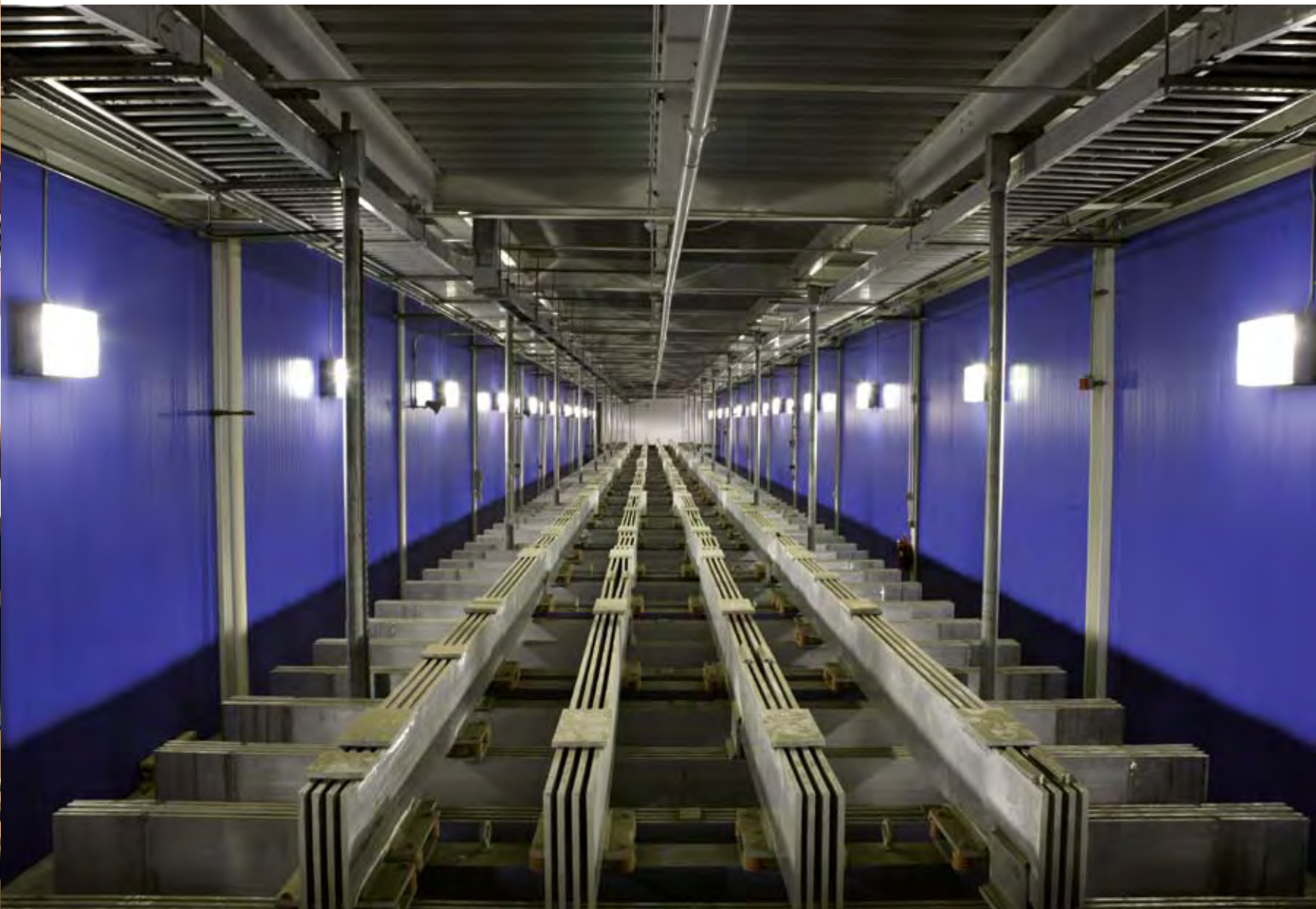
Right: The bus tunnel from end to end. For an idea of how big the room is, see the little dot on the wall at top right? That's a fire alarm box.
