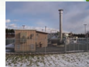
Metering and Regulating Station
