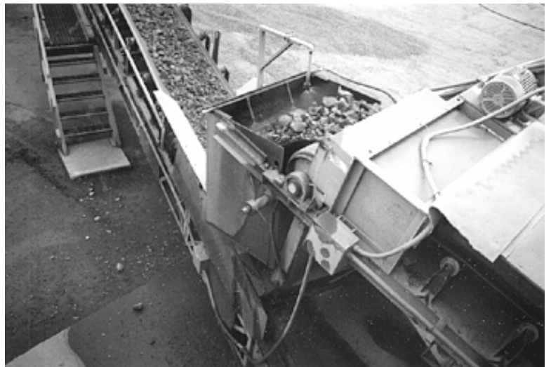
Miners are injured each year by material falling from belt conveyors.
