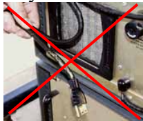
Damaged Cord (exposed wire)
