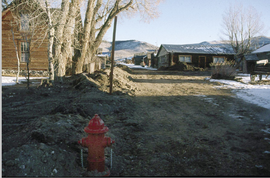
A completed pressure hydrant at the end of a newly filled water line ditch in Virginia City
