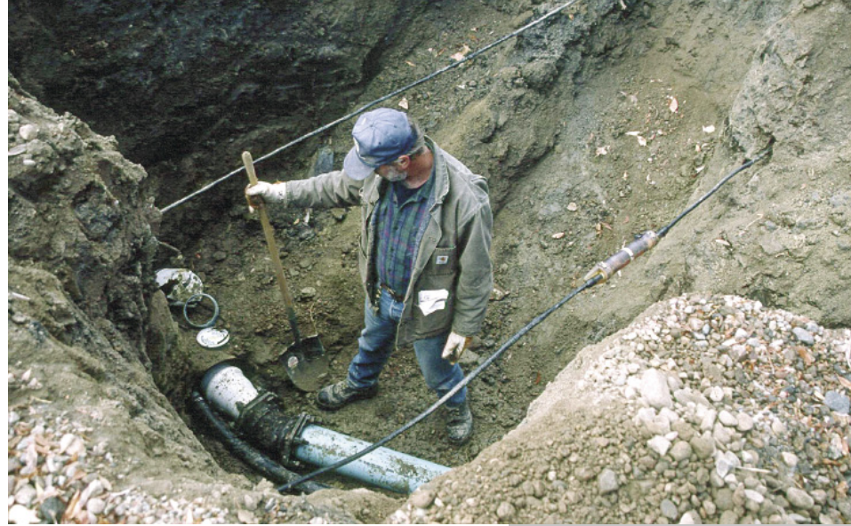
A worker connects the water feeder line to one of the pressure fire hydrants installed in Virginia City
