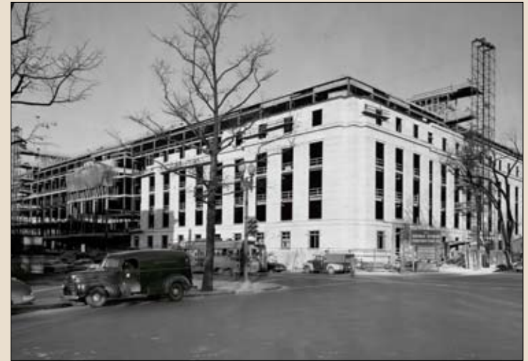
The new Senate Office Building, later named the Dirksen Senate Office Building, under construction in December 1956.
