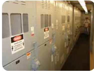
Electrical switch gear
