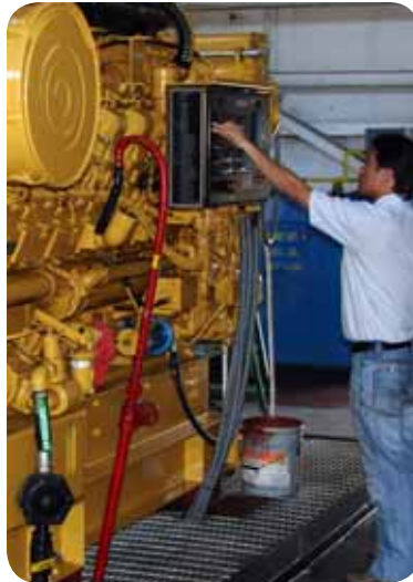
Caterpillar electric generator
