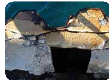
Deteriorated bulkhead on Inner Harbor
