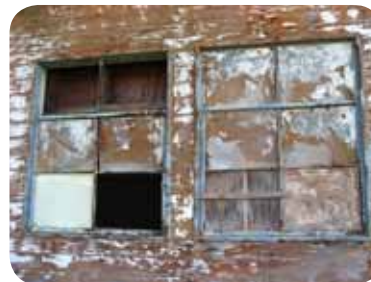
Peeling lead-based paint
