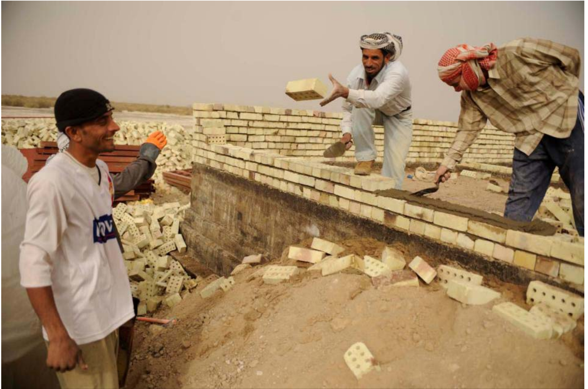
An Iraqi construction worker catches a brick as he and his fellow workers build a school in Budayr, Iraq, Dec. 23, 2008. This is one of three known schools under construction in the Budayr area.
