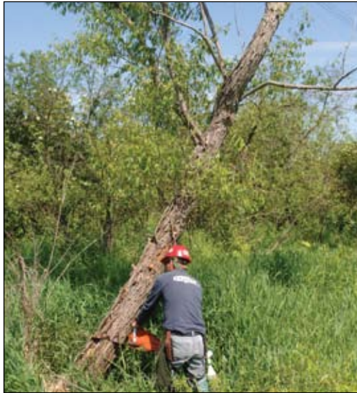
A crew moves into a heavily treed area along a NYPA transmission right of way.
