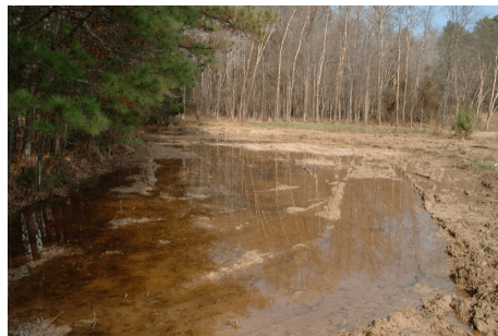
Restoration in progress. Excavation formed crescent-shaped low areas along the field edge in 2001.
