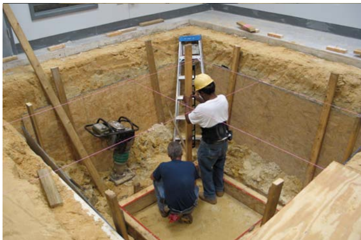
A magnet pit is being readied for the CO-WIN lab, an outgrowth of a $1.5 million grant from the National Nuclear Security Agency to increase the involvement of minority scientists and their students in cutting-edge research.
