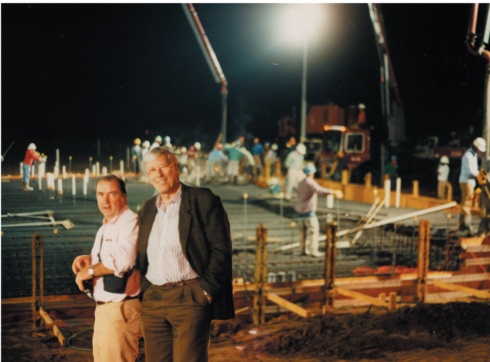
The foundation of the wing housing the user facility with the resistive and hybrid magnets had been designed for maximum stability and low vibrations. The casting of the 1 m thick slab took several days and nights. It was the largest amount of concrete ever poured in Northern Florida.
