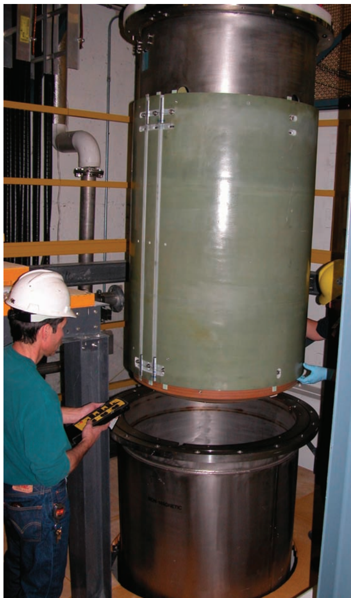
Figure 3. The completed 60TCW being installed in the liquid nitrogen dewar.
