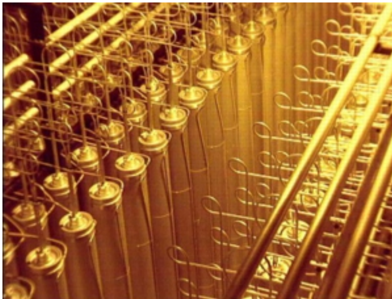
Figure C1-9. Top view of a bank of centrifuges at a URENCO gas centrifuge plant.
