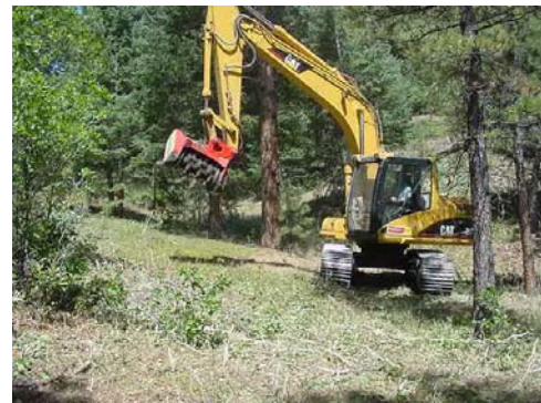
Figure 27. A “Bull Hog” cutting head being used on the South Platte project in Colorado.
