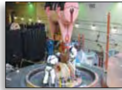
June 1 Upgrade on first of four pump-turbine generating units at Blenheim-Gilboa completed in time for peak summer power demand season.
