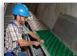
April 4 Power Authority receives award for waterways stewardship for eel ladder installed at the St. Lawrence-FDR project in Massena.
