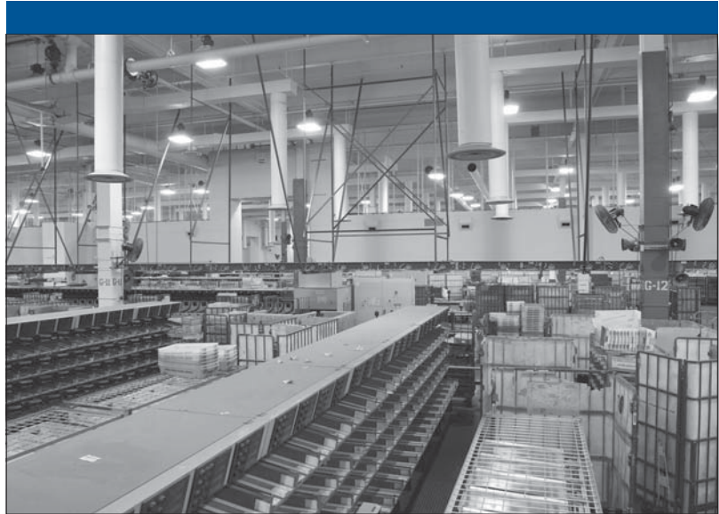
In assessing the Postal Service's energy management strategy, the Office of Audit recommended expanding short-range planning, including more facilities, and updating energy policies to increase its effectiveness.
