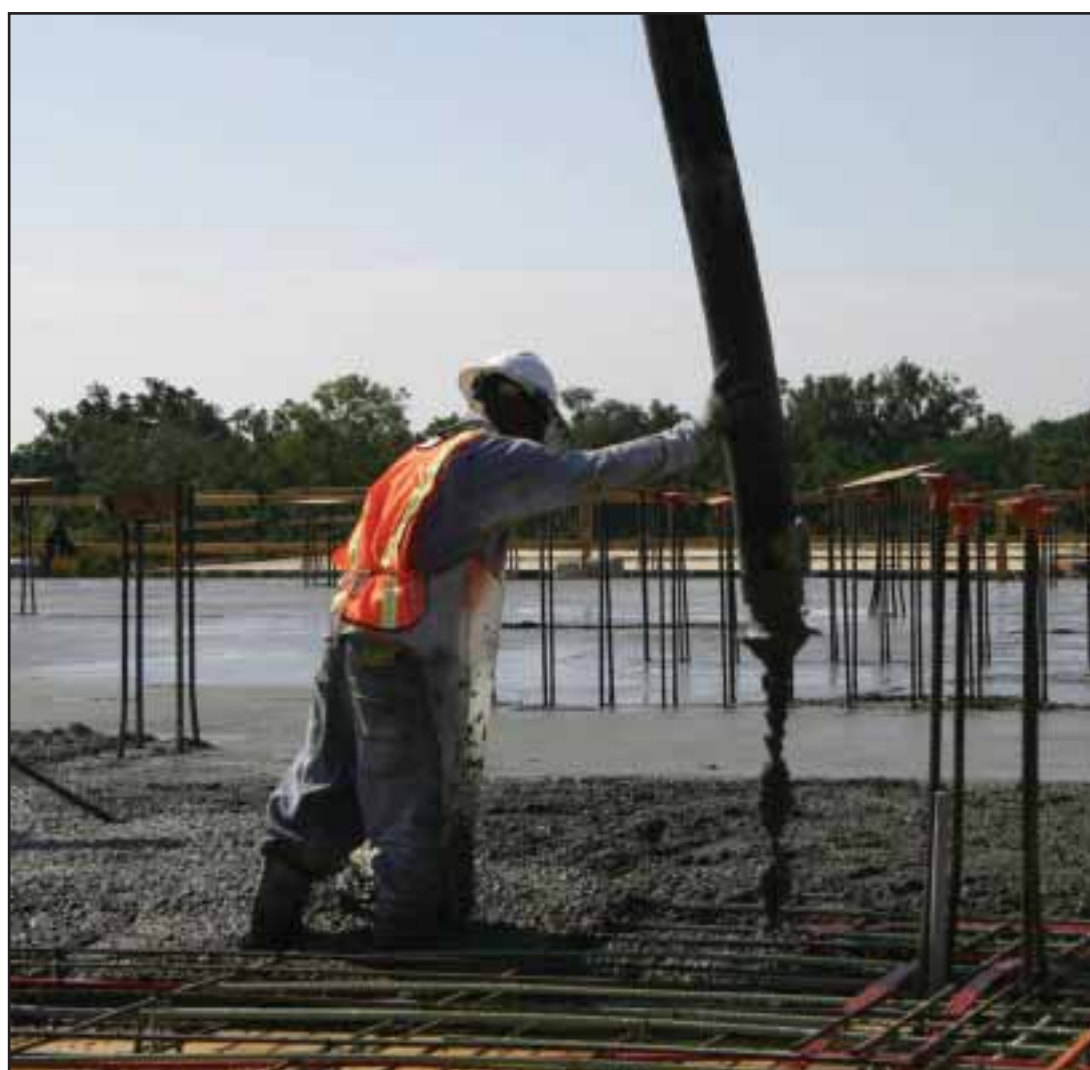
The third deck. As of August 26, 2008 a total of 14,737 cubic yards of concrete have been placed.
