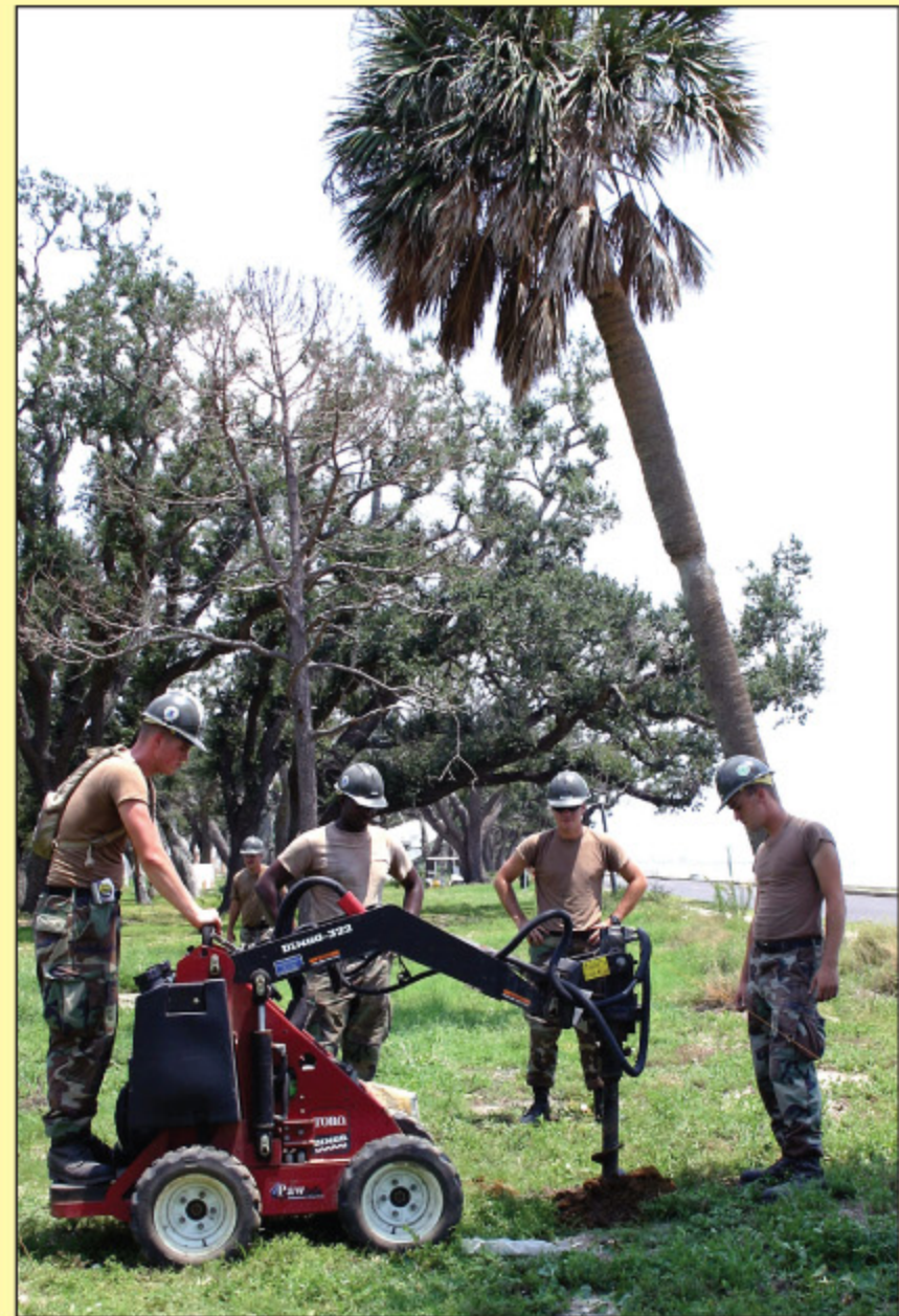
Concentina wire replaced with fence - Seabees from NMCB-74 work out front digging fence post holes. The Seabees replaced the fence that was destroyed from the storm.
