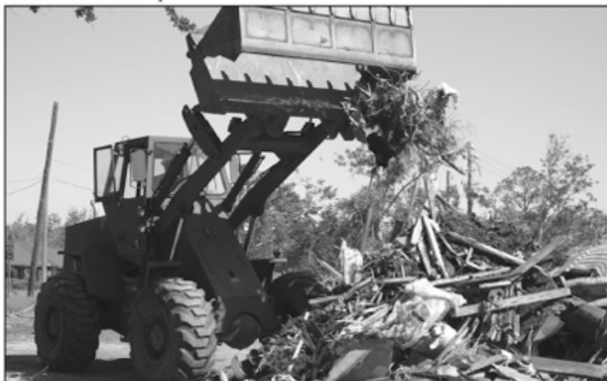
A Navy equipment operator gathers debris into a pile readying it for removal.
