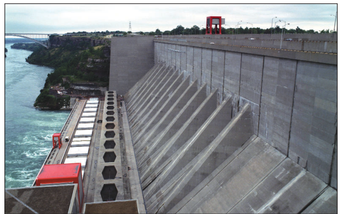
The concrete face of the Robert Moses Niagara Power Plant will undergo repairs during the next three years.
