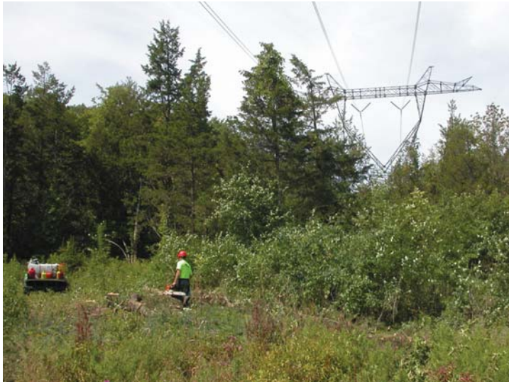
Crews prepare to trim trees growing too near NYPA's high-voltage transmission lines. Several vegetation-control techniques are used.
