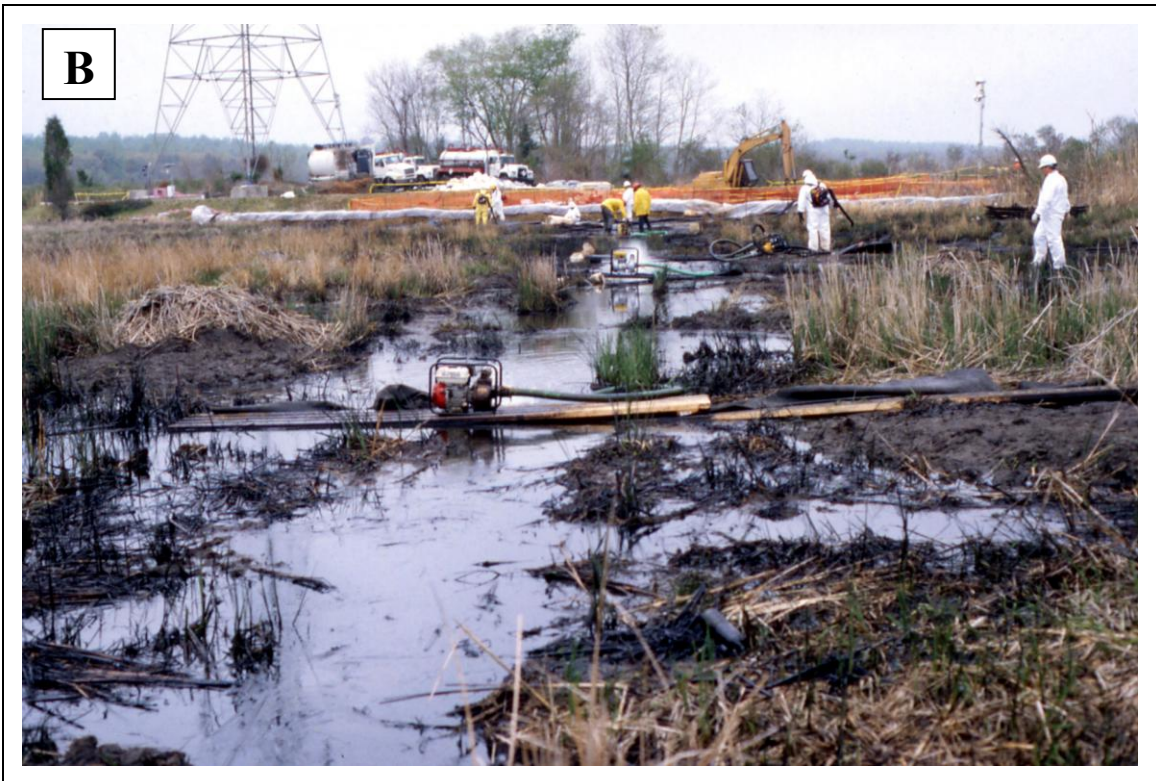
FIGURE 4. A. Cleanup methods used in the marsh adjacent to the leak site, located to the right of and adjacent to the access road. Note the extensive use of trenching. B. Flushing on the ground. The trenches were eventually filled and planted.
