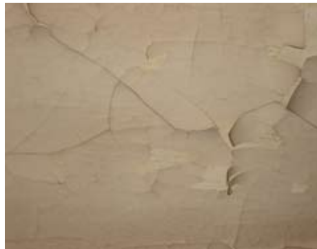
Figure 2: While top paint coats may not contain lead, under layers may have high lead content.
