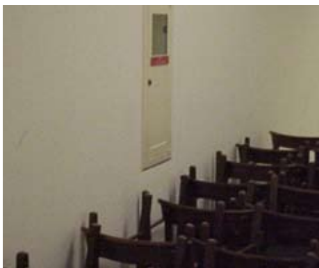
Figure 1: Pull station and Fire Extinguisher Blocked by Stored Furniture in Corridor
