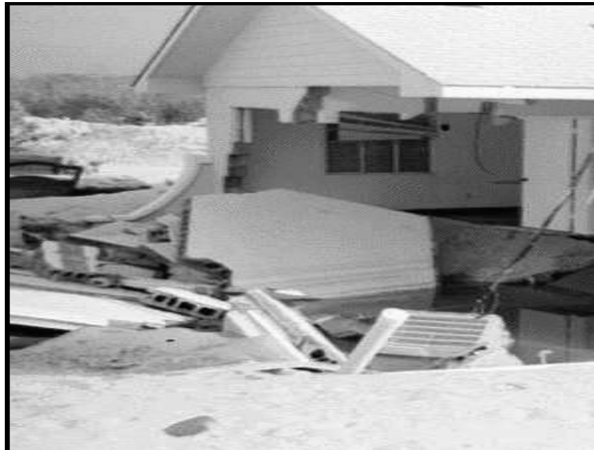
Figure 1-16. Beaches are particularly susceptible to undermining of foundations due to velocity flows.
