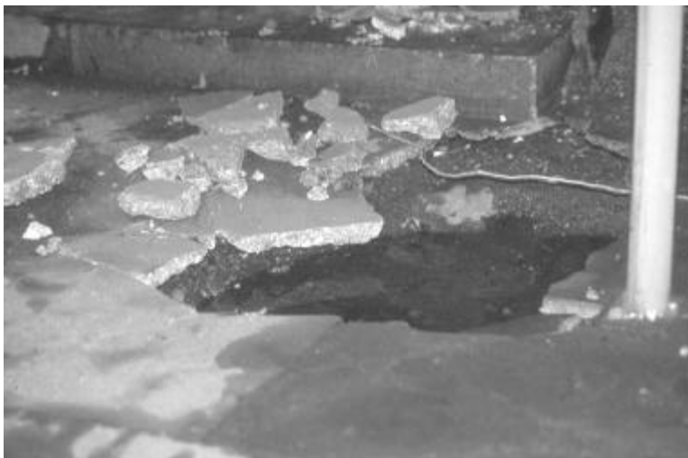
Figure 1-19. This basement floor broke from hydrostatic pressure
