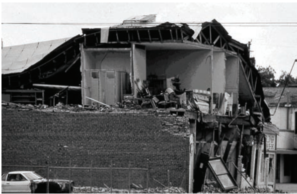
Figure 9-4: Nonstructural partition walls prevented the total collapse of this unreinforced masonry structure in the 1983 Coalinga earthquake.
