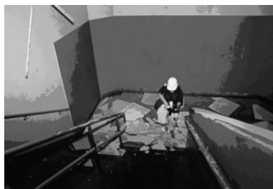
Figure 9-6: Difficulty in exiting due to debris strewn across exit stairs can be an indirect threat to life, as can be seen in this photo following the Loma Prieta earthquake in 1989.
