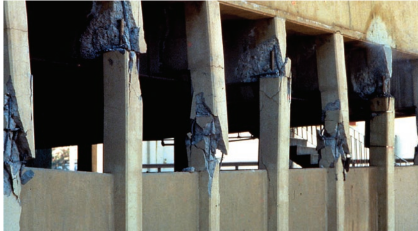
Figure 5-29: Damaged parking structure, Whittier Narrows (Los Angeles) earthquake, 1987. The deep spandrels create a strong-beam, weak-column condition.
