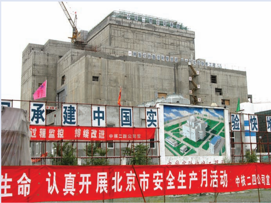
Full steam ahead. Construction is well under way on China's first experimental fast breeder reactor, located in Tuoli.
