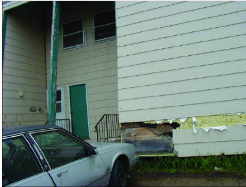
A home on the Turtle Mountain Indian Reservation in North Dakota shows damage caused by the wet environmental conditions in the community. The high moisture levels both indoors and outside are likely the main contributor to CDC's finding that 60% of the homes inspected had visible mold contamination.
